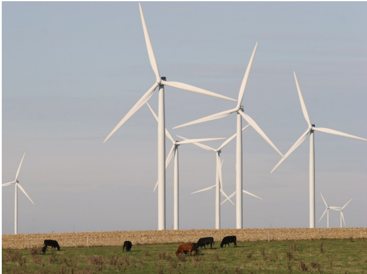
A wind farm in Texas, which leads the U.S. in wind energy production. The U.S. produces more megawatt hours of wind energy than any other nation. Photo: U.S. Department of Commerce
