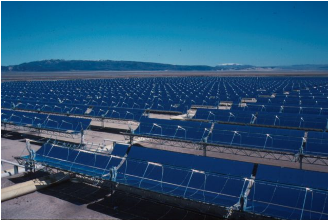
Part of the 354 MW Solar Energy Generating Systems parabolic trough solar complex in northern San Bernardino County, California. Photo: U.S. Bureau of Land Management
